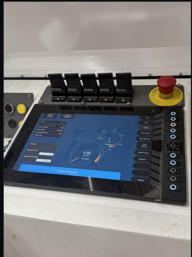
THE SAME CONSOLE ON THE MUD SCREEN — FLOW RATE, PRESSURE AND THE PRESSURE CUT-OFF
