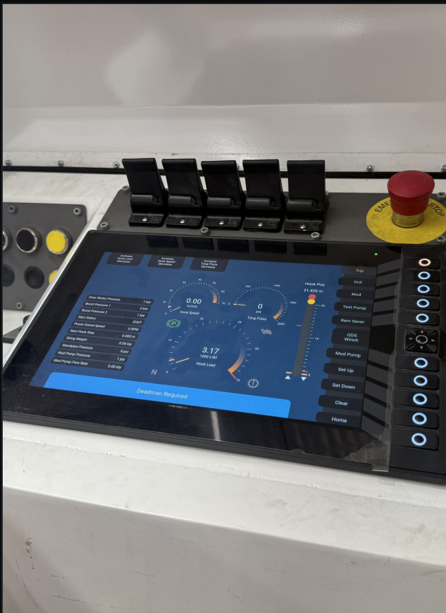
THE CONSOLE RUNNING THE TRIPPING SCREEN — HOOK LOAD, HOOK POSITION AND THE DEADMAN INTERLOCK PROMPT
